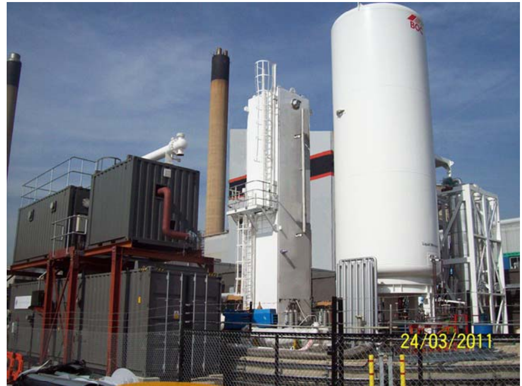
Source: Highview Power Storage
